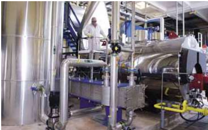
Energy eco-efficiency installation in the Vichy plant.
